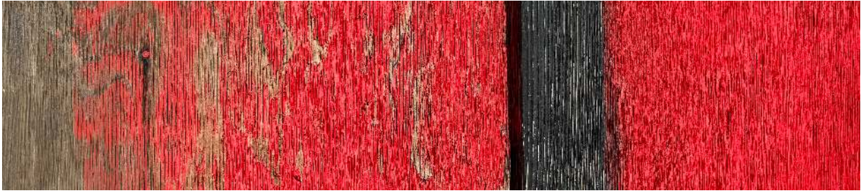
Detail documenting a weathered red-painted wood surface associated with an ancillary building on the south side of the building.
