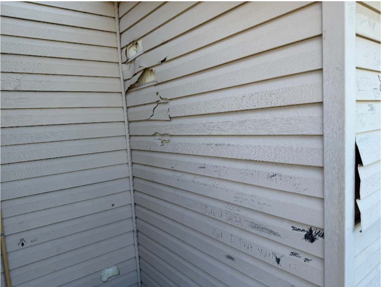
Detail showing the junction between building sections and localized siding damage.
