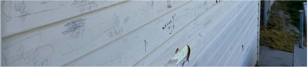
Detail documenting horizontal siding, surface markings, and material condition.
